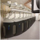
9 biogas fuel cells in container connected to building heating system (and preheated by datacenter)
